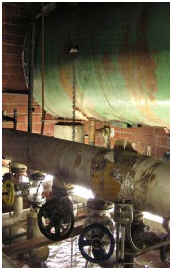
Aging Mechanical Systems
